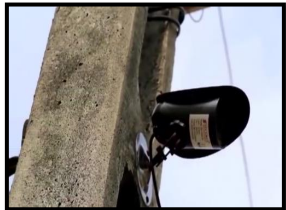
Fig.3.3.6 - CCTV facility in Punsari
