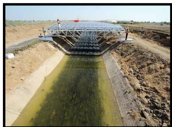
Fig.3.3.3-Solar panels on canal
